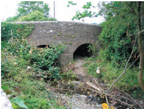
Litter and debris at the stream
