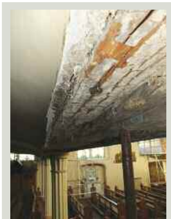
Regular inspections and scheduled maintenance work should prevent rot from taking hold to the degree that it causes structural damage, as has happened to this beam which supports an organ gallery
