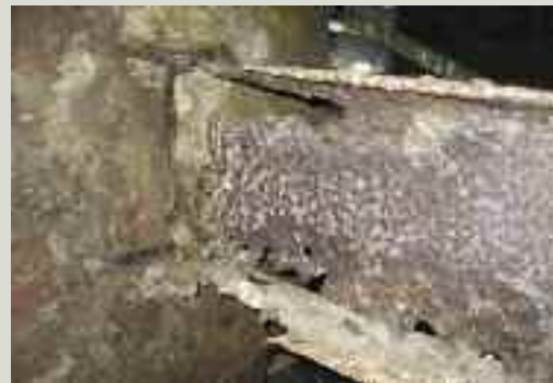
The extent to which driving rain and lack of a protective coating can damage bell supports is shown by this badly corroded steel beam
