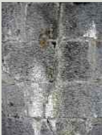
This wall has become overly rigid due to the use of cement mortars, which resulted in the mortar becoming harder than the stone. Structural movement in the church is seen in the vertical cracking through the ashlar stones rather than the mortar
