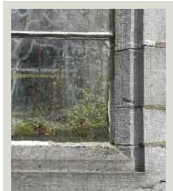
Sealed, or inadequately ventilated, storm glazing provides an opportunity for the growth of vegetation, which damages the stained glass as well as being unsightly
