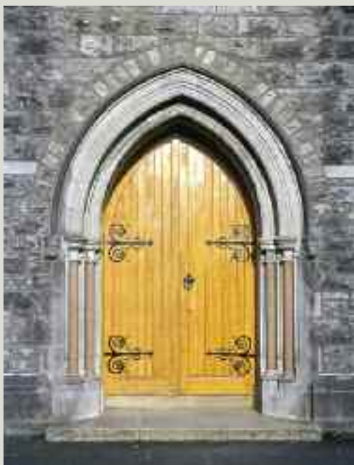
Historic doors and door furniture should be maintained and repaired as necessary in line with best conservation practice
