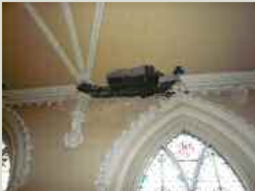
Neglect of the roof of this church led to moisture ingress and timber decay, resulting in serious damage to decorative plasterwork. Investigations determined the extent of the problem, which was remedied using traditional plaster repair methods and the removal of as little structural timber as necessary
