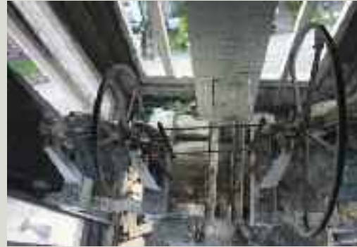
This belfry was photographed prior to work commencing on the steeple (but after the louvres were removed to provide more light for the duration of the project). In common with all such areas, the signs of pigeon infestation are everywhere, however the structure and bell mechanism are in a reasonable condition
