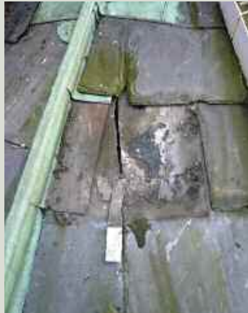
A previously repaired slate slipped off this chancel roof (the clip or tingle remains), revealing a hole in the covering and leaving some of the copper flashing vulnerable to uplift
