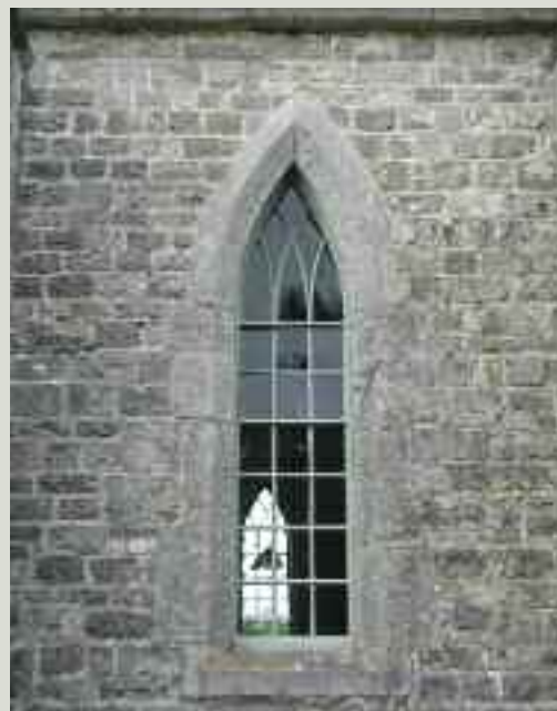
The simple iron glazing in the lancet windows of this rural Board of First Fruits church is enhanced greatly by the survival of crown and cylinder glass. The windows, and the church, are clearly well cared for
