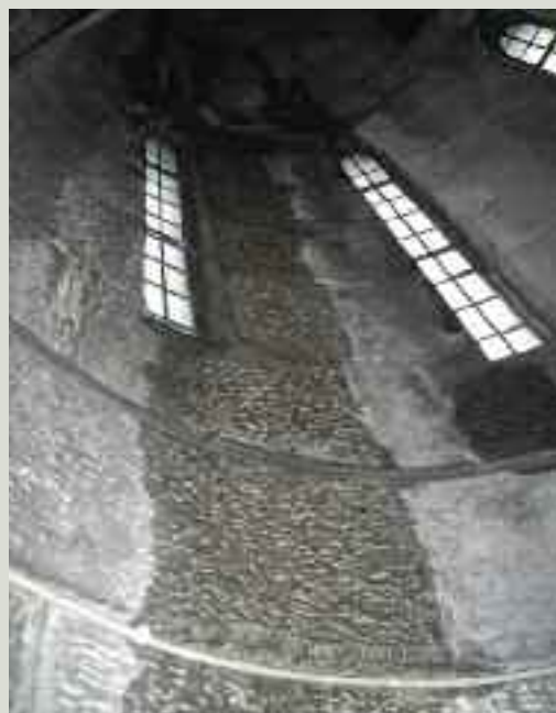
Difficulty of access no doubt contributed to lack of maintenance of this church tower, resulting in ingress of water to saturation level in the masonry. This will lead inevitably to serious damage unless it is remedied
